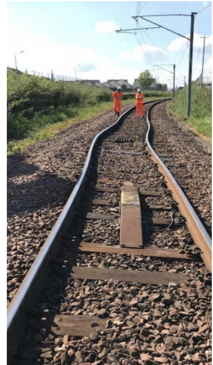
Lines near Glasgow buckled due to heat, June 2018. Image credit: Network Rail
